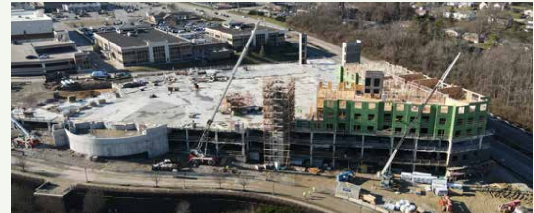
Work continues at the Vantage at Anderson Towne Center Apartments and park and ride project on Five Mile Road.
