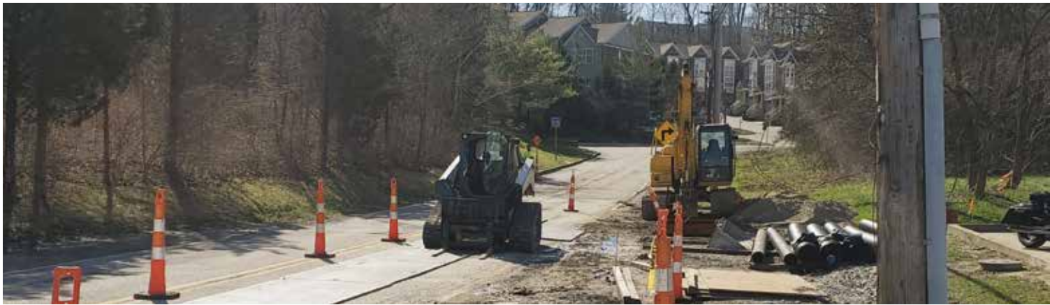
The new Elstun Connector, pictured here under construction, will link the Skytop area to several regional trails.
